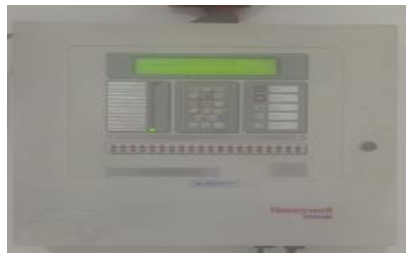
HLL Installed with 03 Fire Alarm Panels in Block A-B & Unit-II with 40 MCPs
